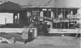
THIS NEW Gasoline pump house office, being built next to the old building for the Process Department, will provide facilities for supervision of loading of all clean oil that leaves the area for producing lead-free fuels.
